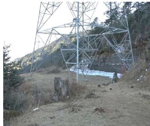
Transmission tower erected on Govt. land without lease
