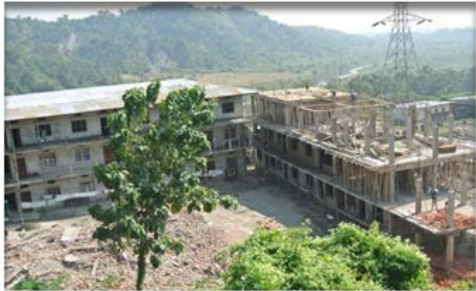
Encroached land used for constructing staff colony by SD FerroSiliconat Matanga
