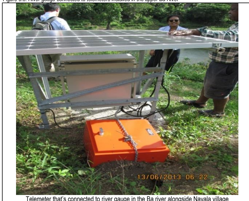
Figure 5.3: River gauge connected to telemeters installed in the upper Ba River
