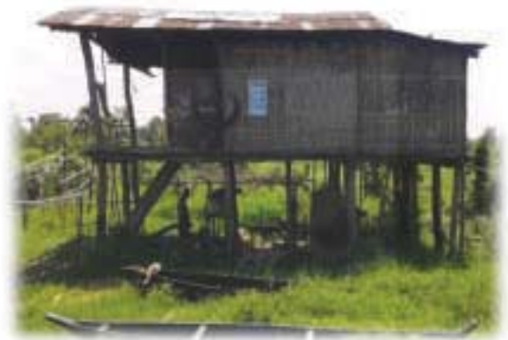
Some of the anti-poaching camps needing immediate repair.
