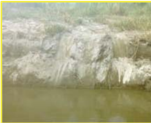
Erosion on the north bank of KNP by river Brahmaputra
