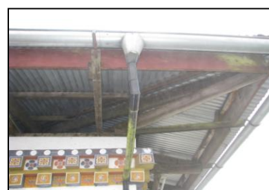
Rain water harvesting at Yongla
