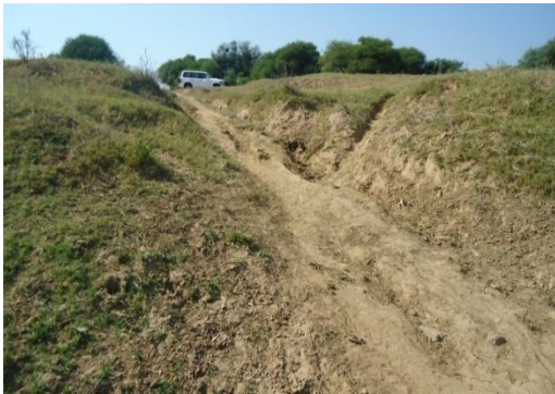
Figure 9 An access ramp that had not been restored along Metsimothabe River
