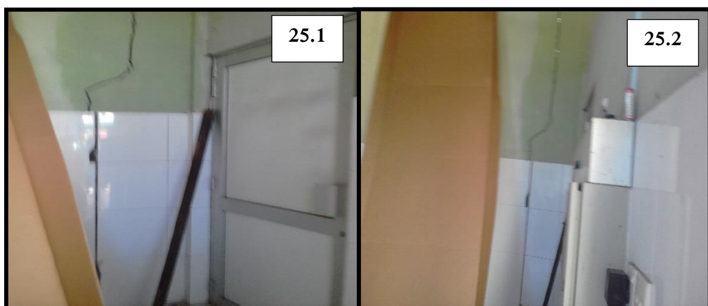
The cracked wall
