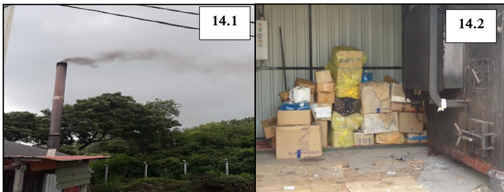
Incinerator at Trincomalee Hospital
