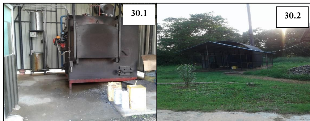
Incinerator at Kanthale Hospital
