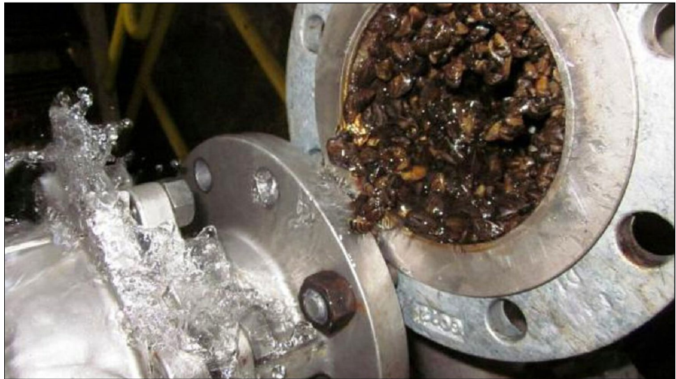
Figure 2: Zebra Mussels Clogging a Pipe
