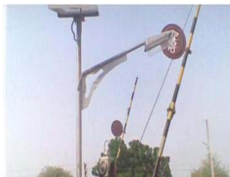
Solar Panel at manned level crossing between Darazpur - Mustafabad section, NR
