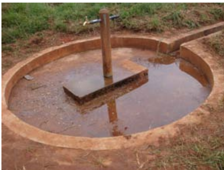
Standpipe in a school in Kilolo - Tanzania
