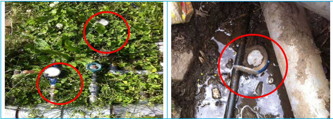
Figure No. 13: Inappropriate water meter installation
