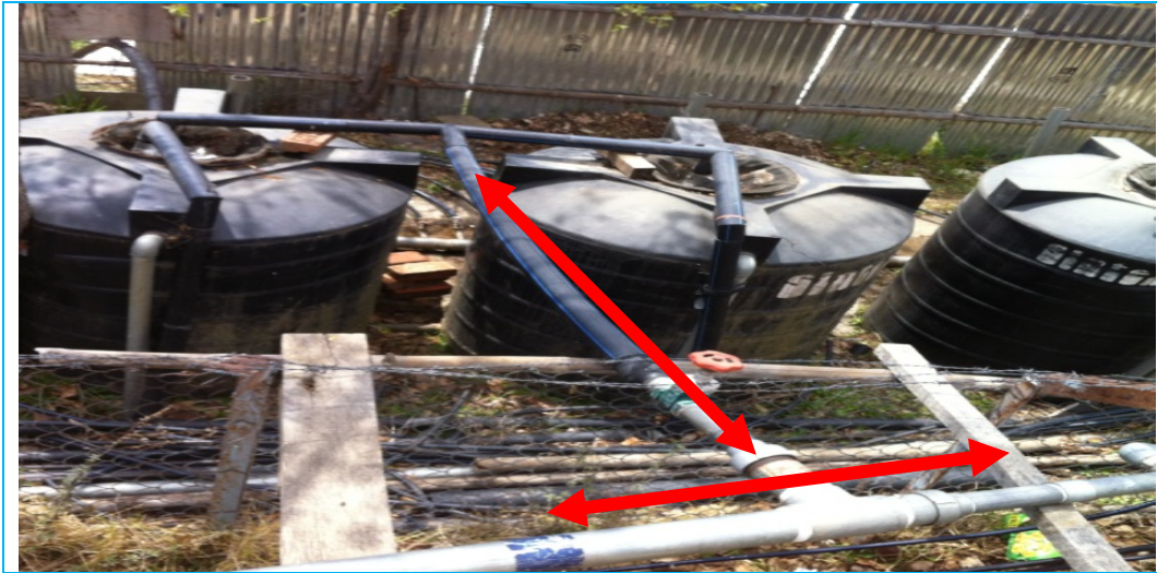
Figure: 7: Connection from transmission line (Changjalu community tank)
