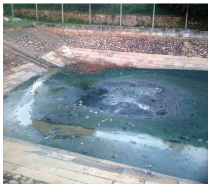
Sections of the Hoima ponds filled with sludge.
