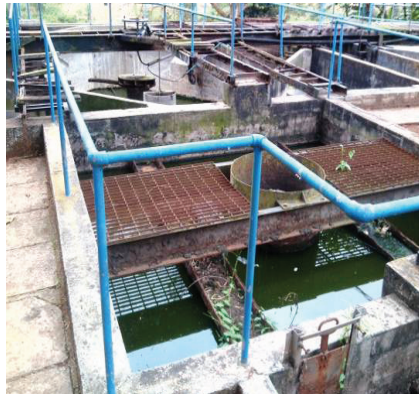
Sections of the Masaka plant were visually rusty and some parts were broken
