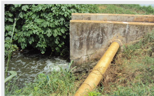
Picture 2 - Direct flow of wastewater still under treatment into Lake Victoria at Kirinya Sewerage treatment plant due to broken pipe leading wastewater to the nearby wetland for further natural treatment.
