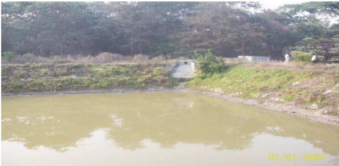
Non functional STP at Halilshar
