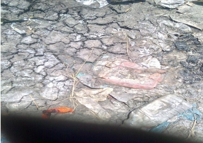
Accumulation of Slit in the Drains and other waste
