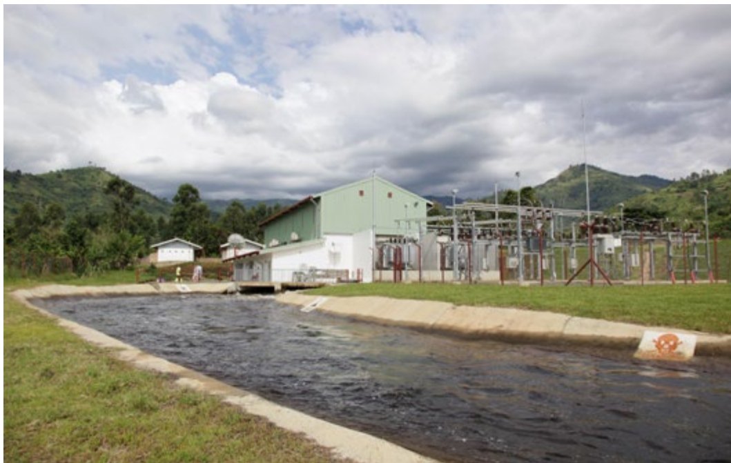
The 13 MW Bugoye hydropower plant in Uganda is one of two power plants that Norfund has invested in in the core countries.
