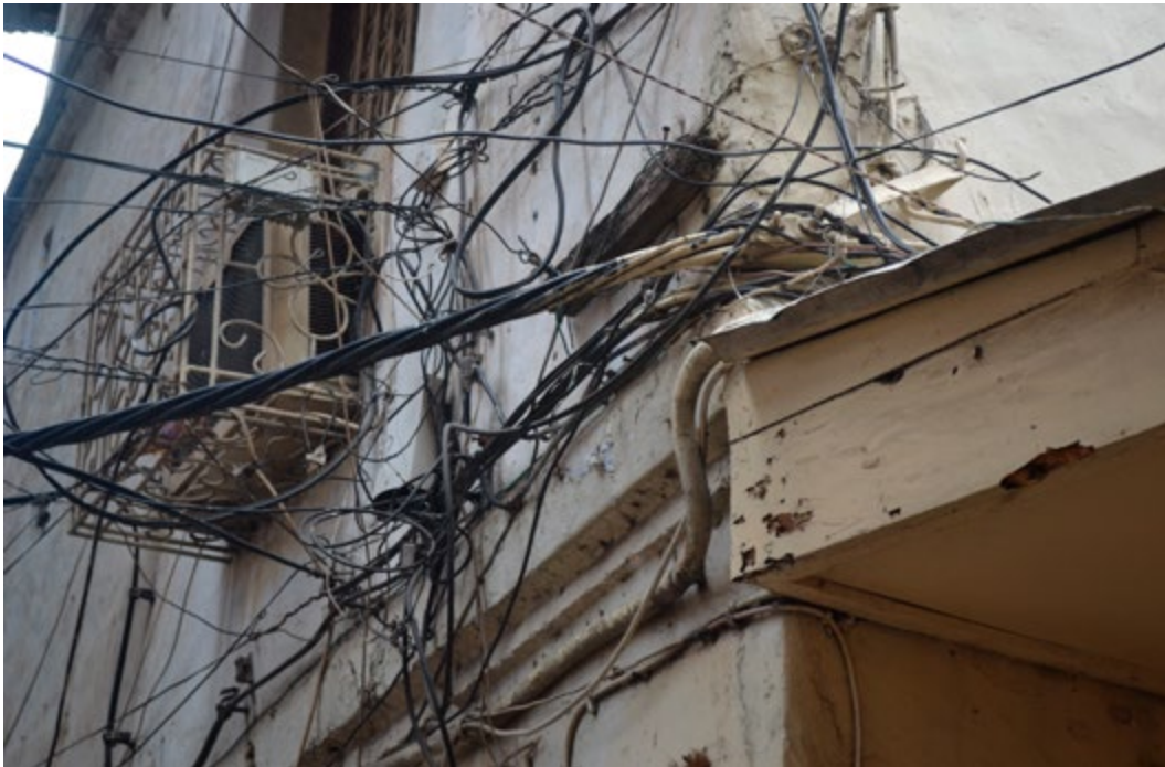
Power lines in Stone Town on Zanzibar.
