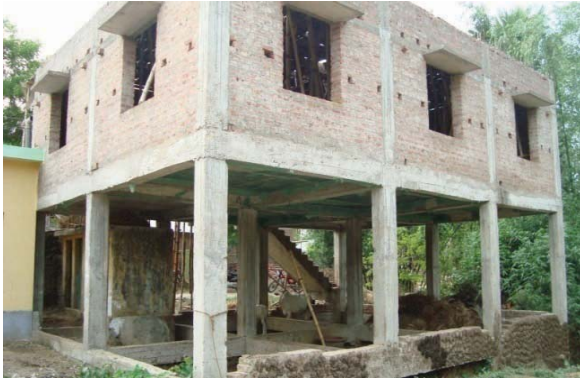
Flood shelter at Dainhat, Katwa-II, Burdwan lying incomplete due to lack of funds
