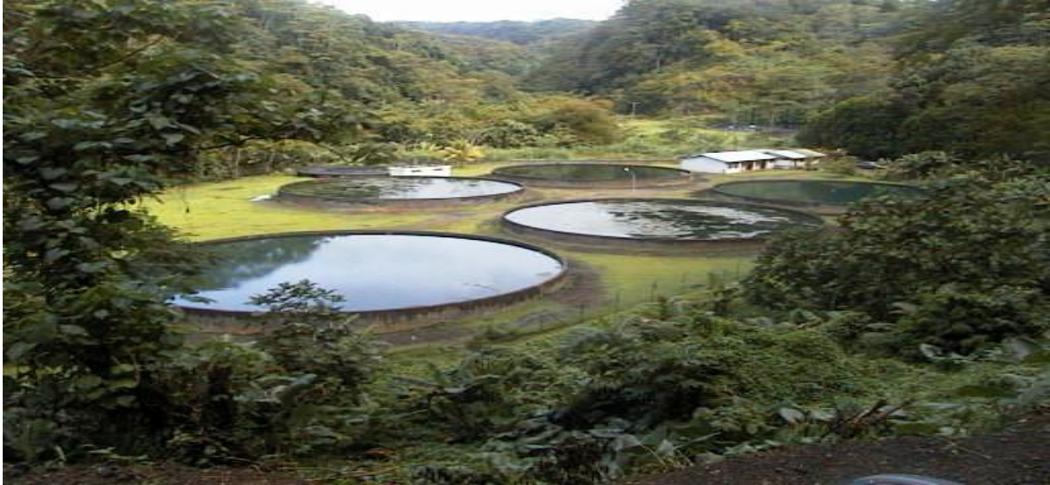
Figure 2: Alaoa Treatment Plant
