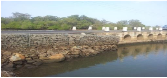
Photograph No 03 -. Bridge blocking sand transport
