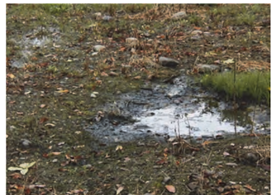
Pooling of domestic wastewater from failing onsite system. Photo: South East Water.
